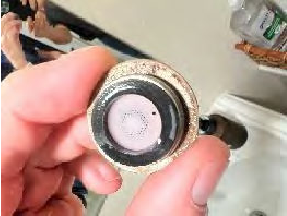
• Photograph 1: Interior of bathroom faucet aerator, with a small black particle and orange colored rust on the perimeter of the aerator surface
