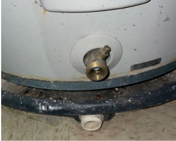
Figure 3. Mild corrosion around the base of the water heater.
